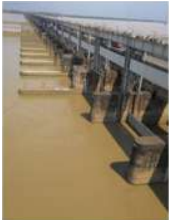
Figure 12. The 2,245 m long Farakka Barrage with 109 gates, 18.30 span, and 76,500 cumecs discharge capacity upon the Ganges (courtesy of SANDRP – South Asia Network on Dams, Rivers and People) Thakkar (2017).
