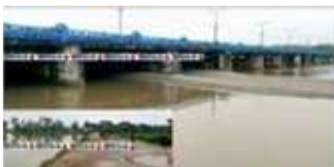
Figure 39. Silts clogged the Teesta Barrage gates Source: The Daily Janakantha, Staff reporter, July 18, 2020). https://www.dhakatribune.com/bangladesh/319168/teesta-flowing-above-danger-level-all-barrage
