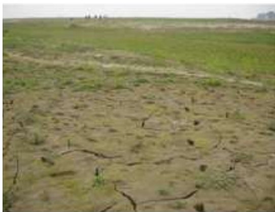
Figure 22. Cracked bed of the Ganges in Rajshahi]. Source: Katz (2008).
